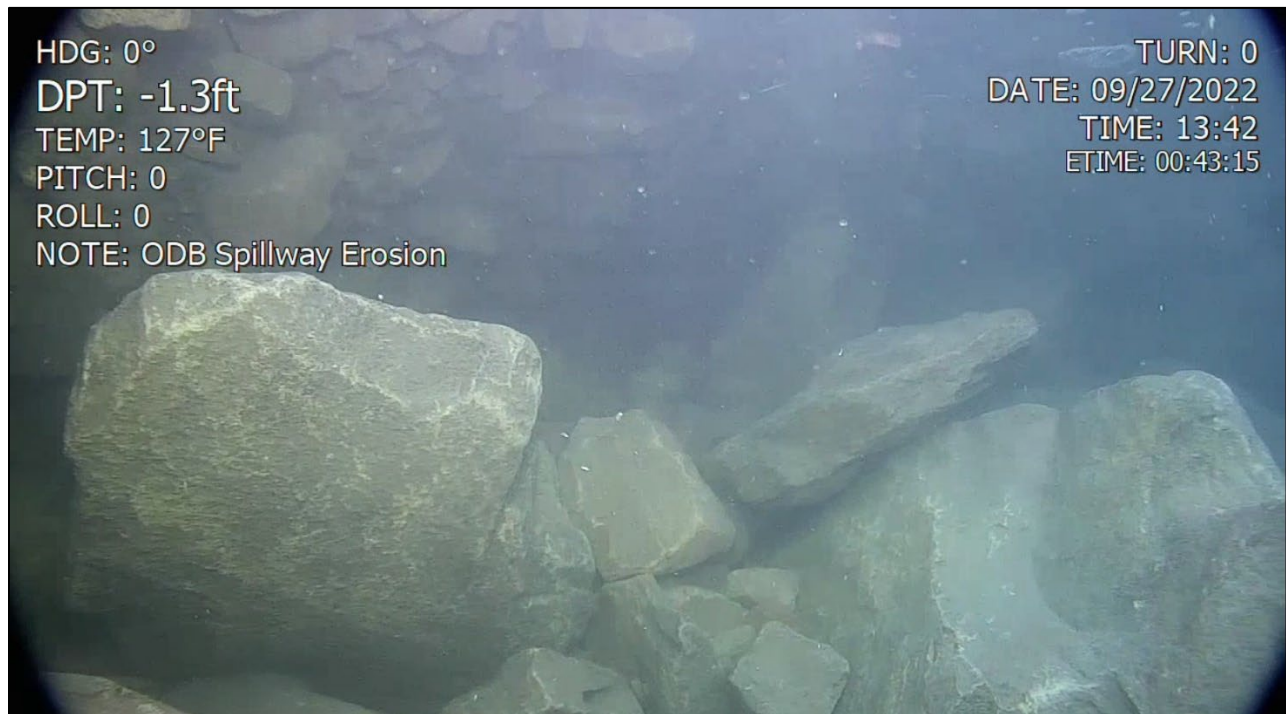
Figure 4 Additional image showing undercut in the southeast corner.
