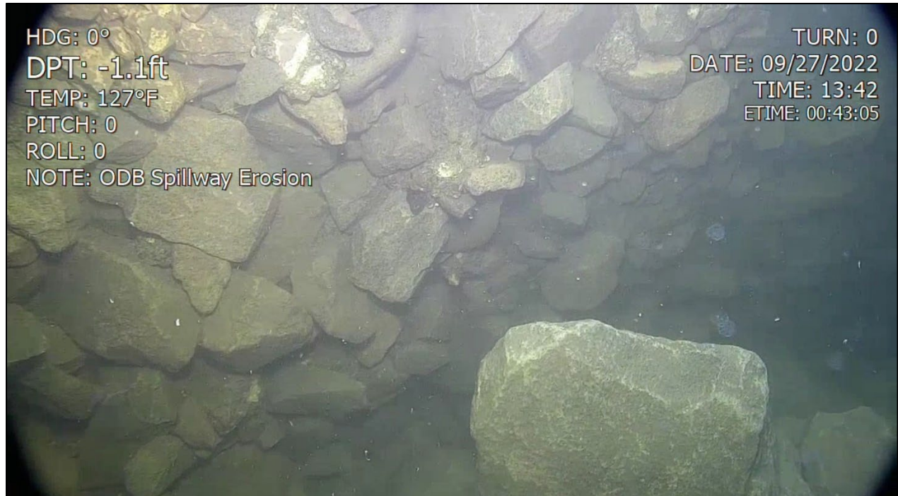
Figure 3 Image of undercut area in the southeast corner of the scour area.
