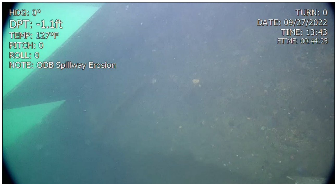
Figure 6 Image showing missing rip rap along western edge of concrete structure.
